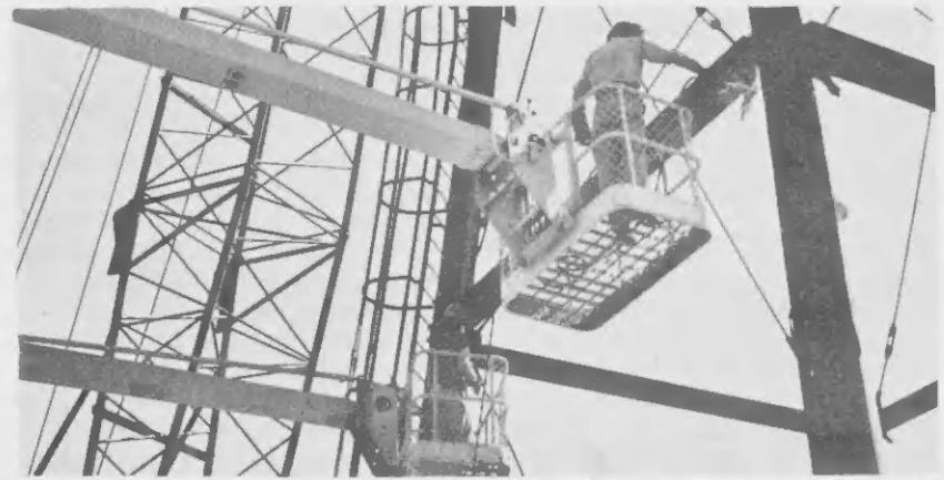
GIRAFFES LIFTED the men with the cutting torches to the designated height at which the legs were to be cut. APARATO DI tipo giraf a hiza e hombernan cu nan torcha di corta na e altura necesario na unda e pianan mester a worde cortá.
